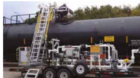
Transloading skid used to transfer product from rail cars direct to road tankers with no intermediate storage facility
