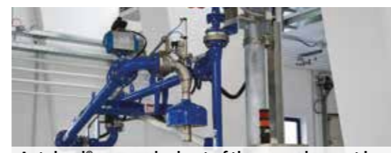
Autoload® arm parked out of the way when not in use. Italy - Chemical industry
