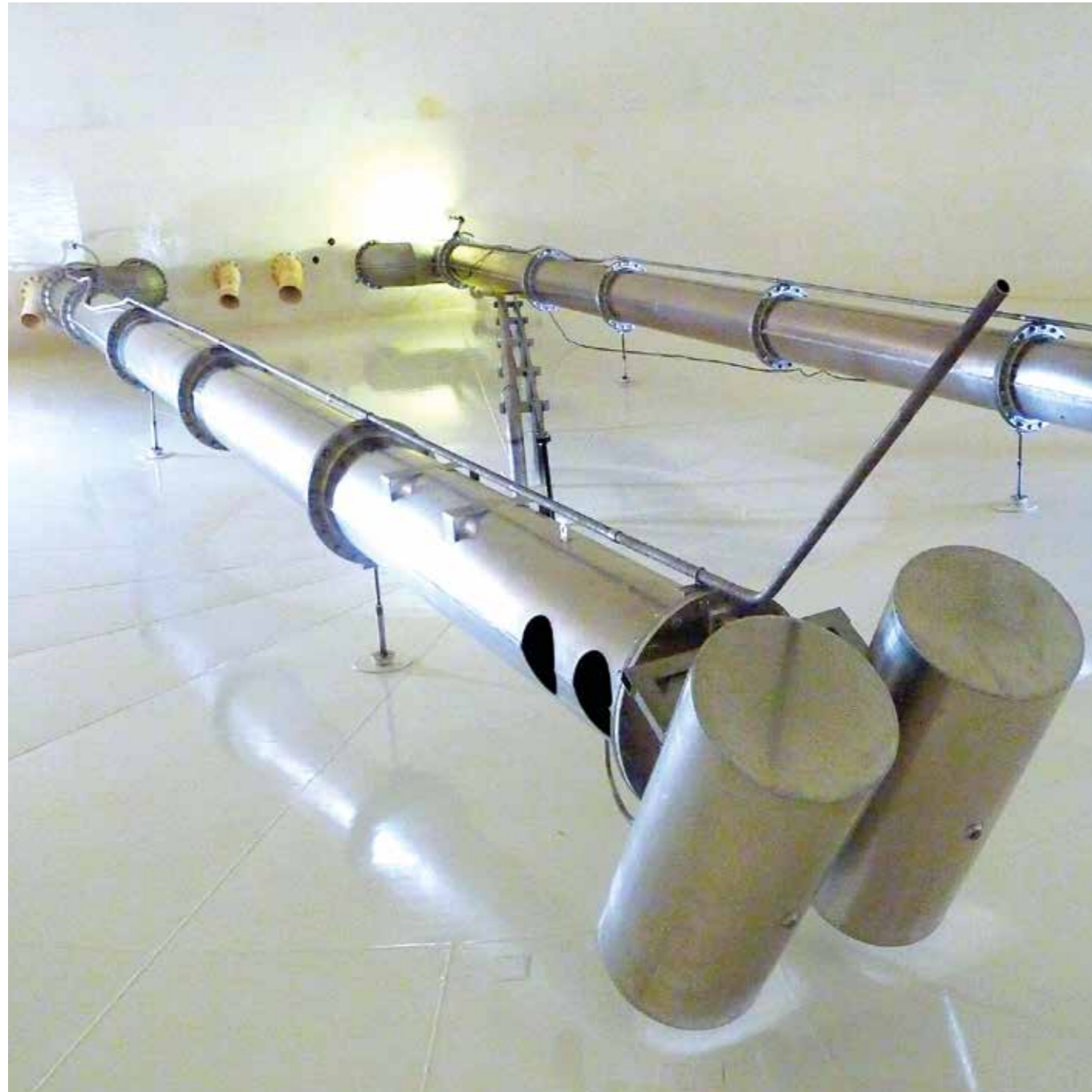
2 x 20" x 15m long Stainless Steel Floating Suctions inside a storage tank ready for Jet Fuel - UK - Aviation
