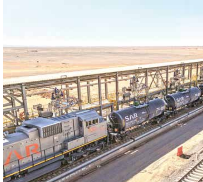
Track mounted Gangways with Loading Arm and meter skids for Acid - Saudi Arabia - Chemical Industry
