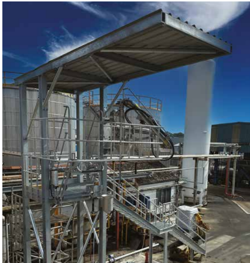
Tanker Loading Platform with Canopy and Loading Arm
