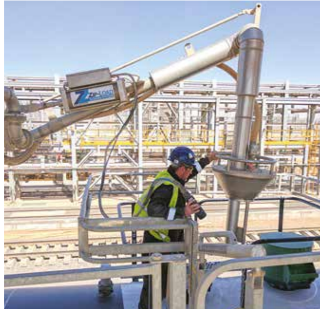
Pneumatic Top loading arm being used inside folding stair Halo cage for rail car loading - Saudi Arabia - Chemical Industry
