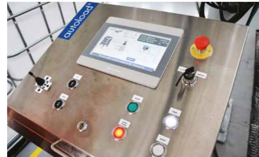
Example of a control panel for the Autoload® arm
