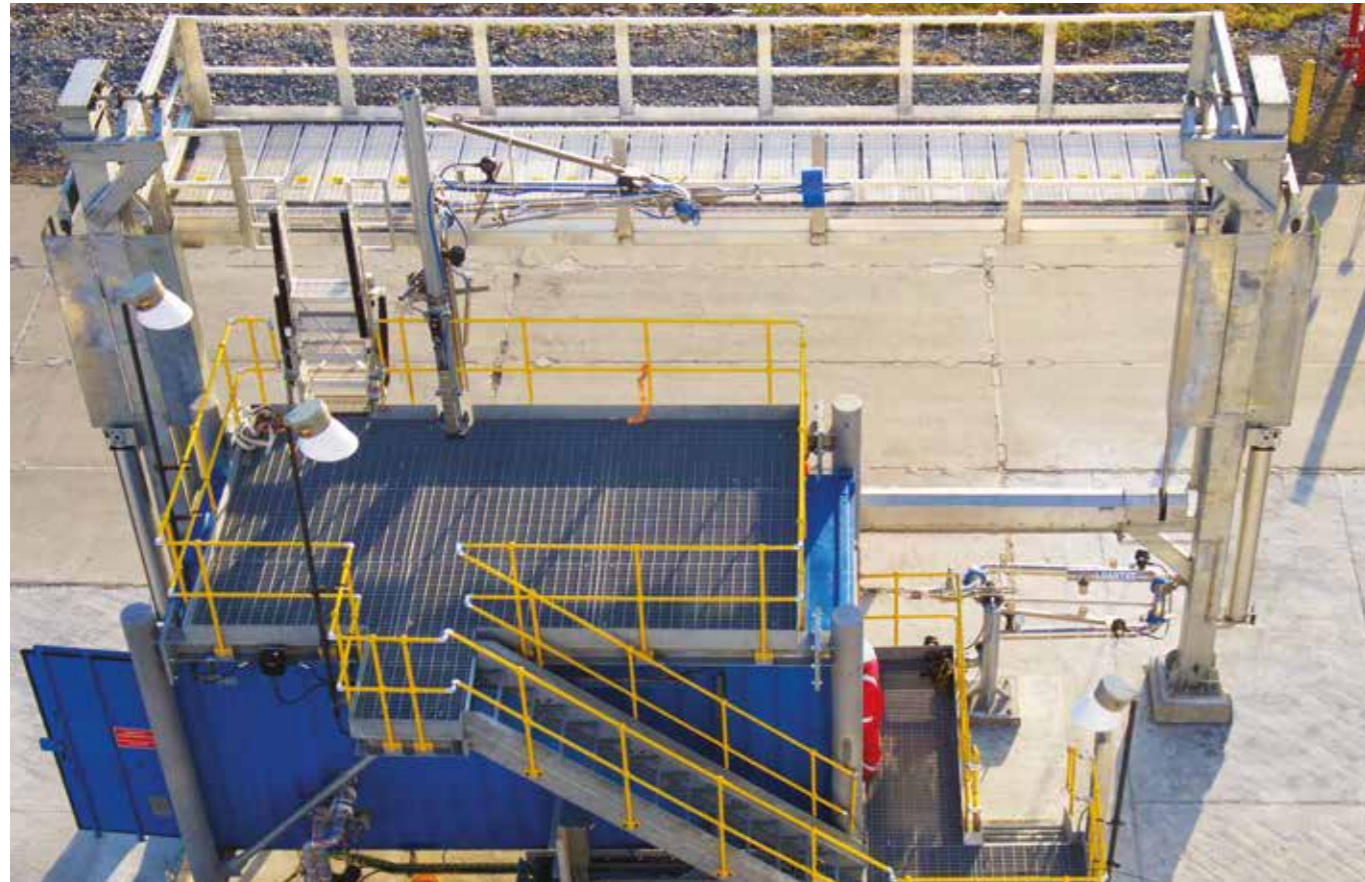
10m VELP pneumatically powered, with top loading and bottom unloading arms, with duty and standby metering skid built into weather proof container subject to extreme sub-zero temperatures. Loading and unloading Artic Diesel in remote locations. Russia- Fuel industry
