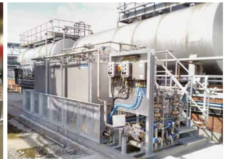
Additive Injection skid with duty and standby metering - UK - Fuels Industry
