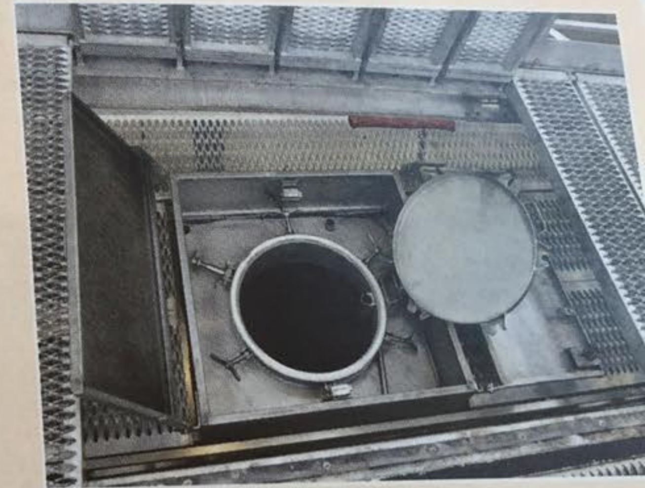
NBO WANTED A COVER TO PREVENT DEBRIS FROM ENTERING THE OPEN MANHOLE
